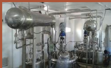
Pharmaceutical GMP Plant
